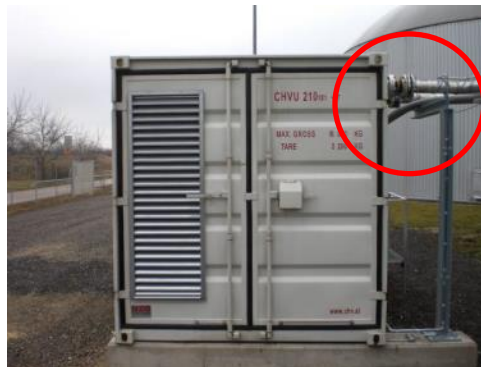
Containerised upgrading unit (membrane)
