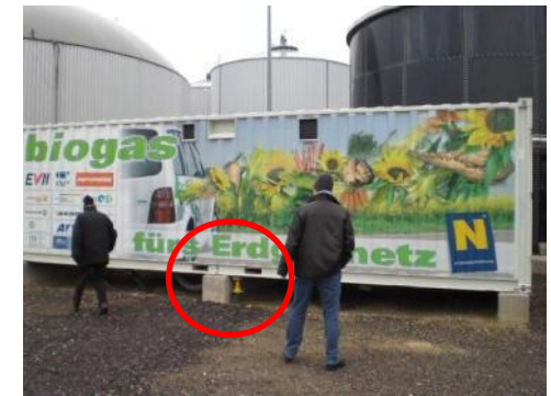
Injection to gas grid
