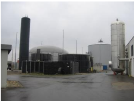
Centralised AD plant
