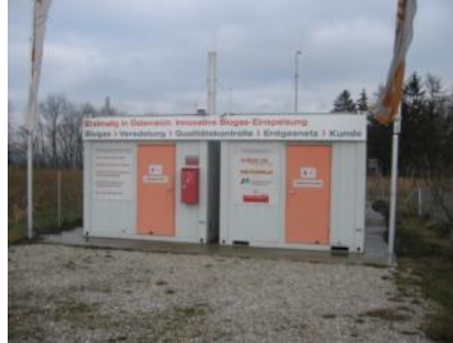
Containerised upgrading unit
