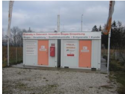
Containerised upgrading unit
